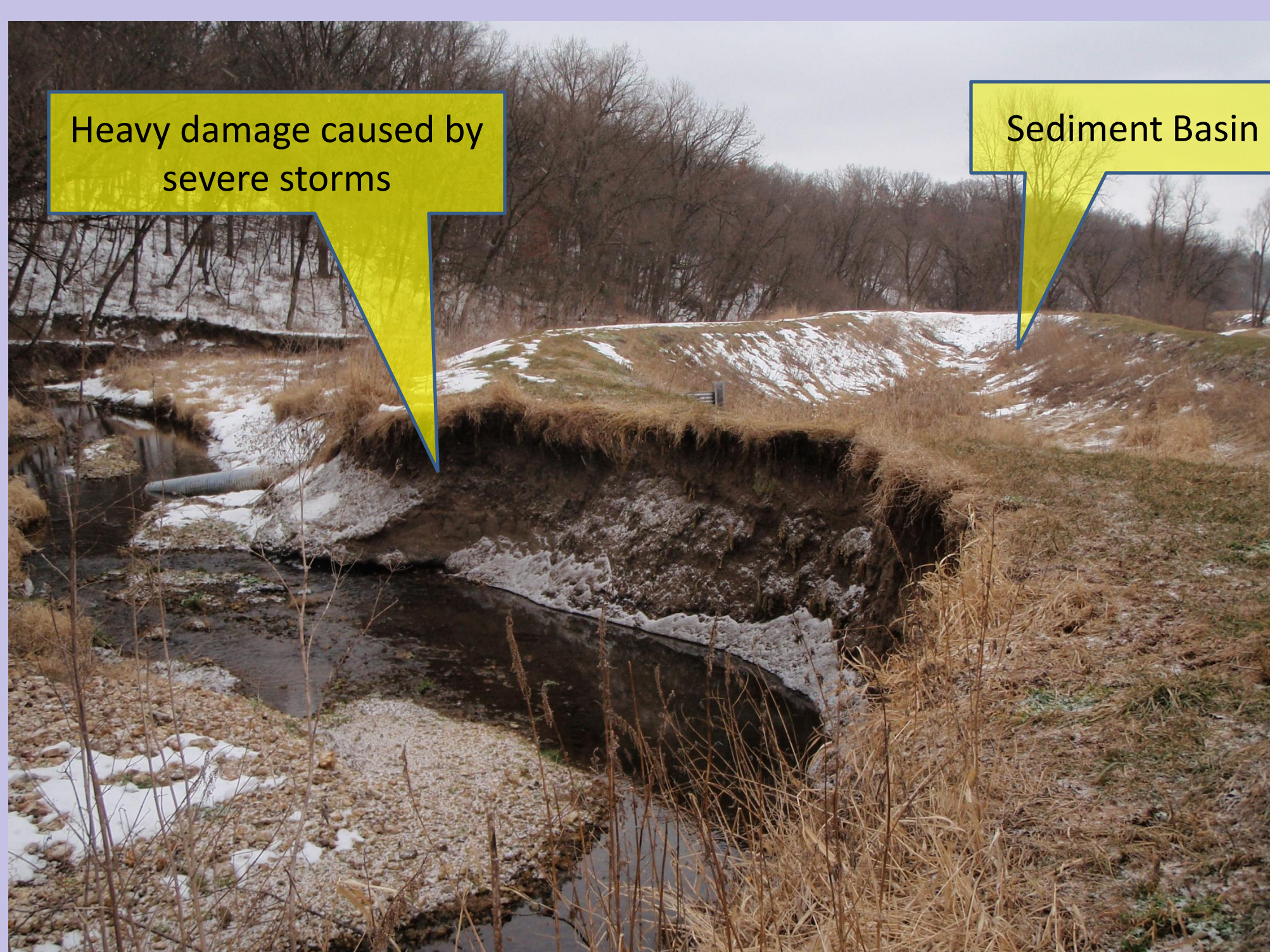
Looking downstream showing stream bank erosion and damage to water and sediment basin infrastructure.
