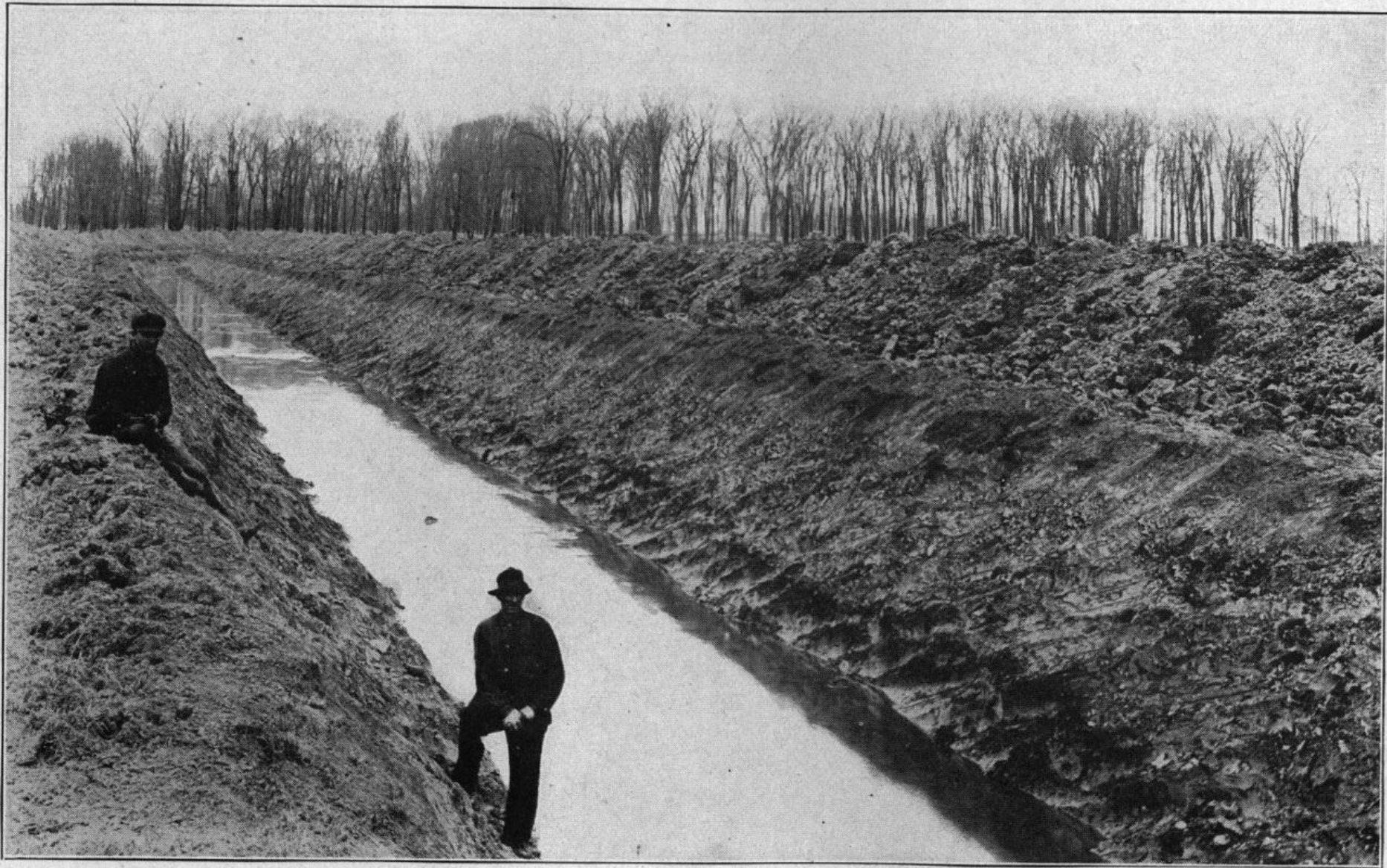
DRAIN EIGHT FEET BOTTOM WIDTH, EIGHT AND ONE-HALF FEET DEEP, CONSTRUCTED BY DREDGE SHOWN IN PLATE V, IN 1917, AT COST OF $7.25 PER ROD (ABOUT \$.08\frac{1}{2} PER CUBIC YARD) TO REPLACE SHALLOW TEAM AND SCRAPER DRAIN CONSTRUCTED IN 1914 AT A COST OF $1.00 PER ROD.
