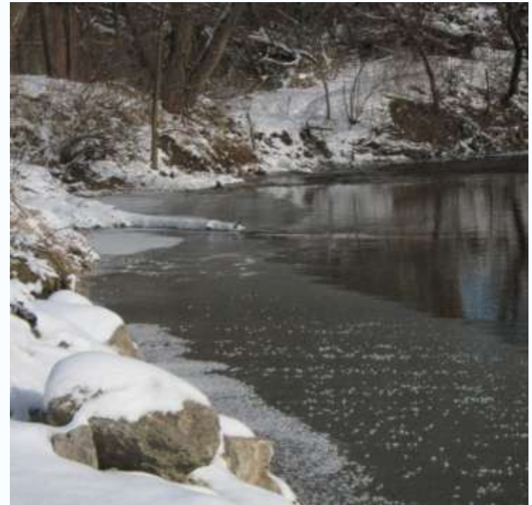
Photo. Ice formation within the backwater of a log vane installed as part of a Brownfield remediation and wastewater pipeline protection project.
