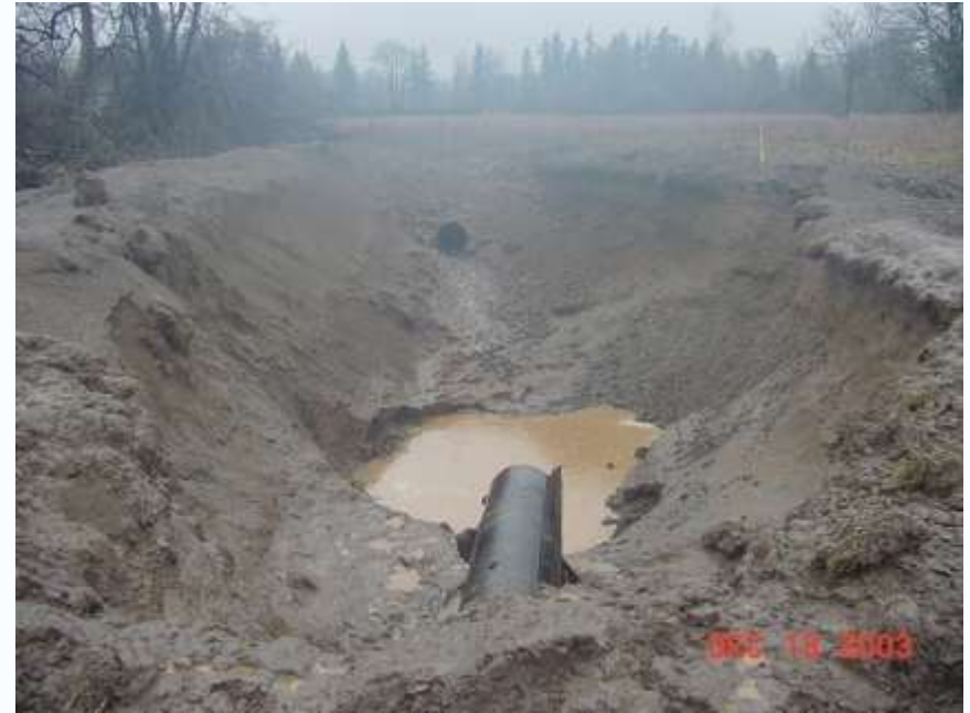
Photo. Ruptured pipeline in rural Washington state. Photo from Washington UTC.
