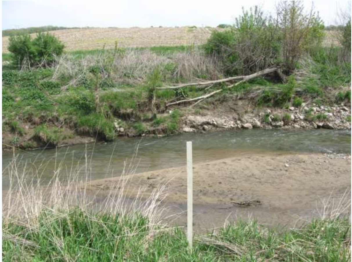
Photo. View across the channel where a pipeline is exposed.
