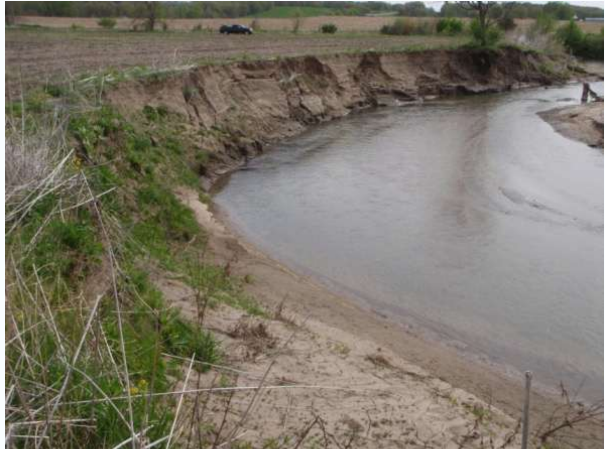
Photo. View downstream at Mill Creek and pipeline area threatened by erosion.
